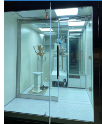
Negative 8Pa Pressured Room
