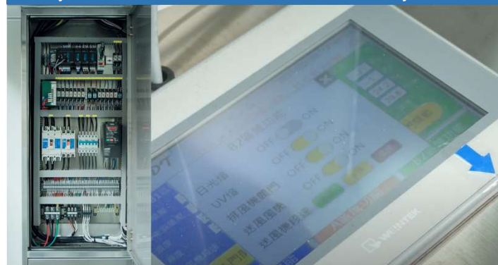
Fully Automated Indoor Environmental Quality Control
